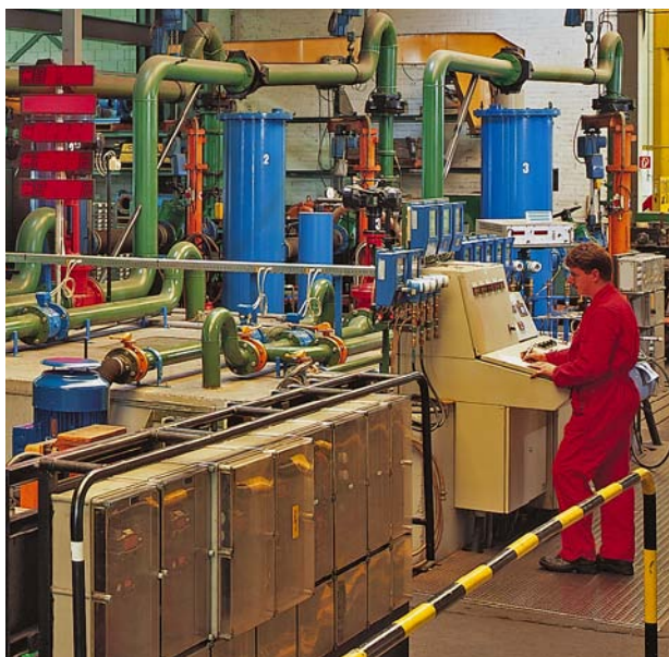
Test bed SPX Flow Technology in Assen, the Netherlands
